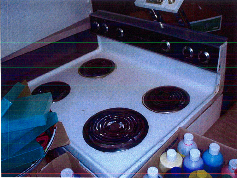
Electric Stove Condition - Fair
