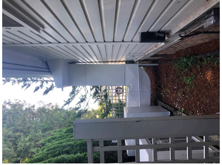
VIEW LOOKING SOUTH AND NORTH FROM WITHIN THE AREA OF THE ADDITION
